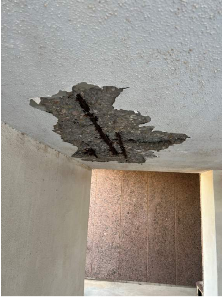
Photograph 9 – Damaged and delaminated concrete on underside of slab at west entry.
