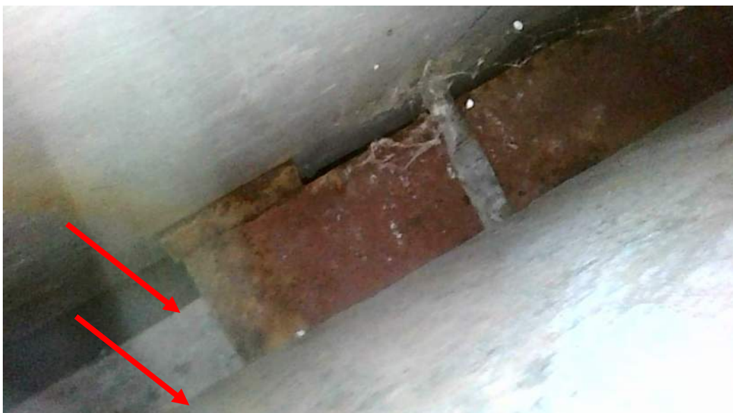
Photograph 6 – Connection at top of displaced granite panel on south elevation with offset in stone.
