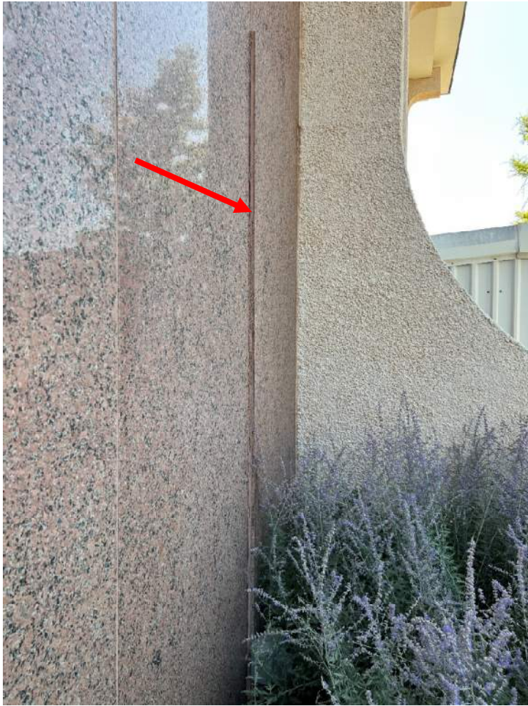
Photograph 5 – Approximate 1 1/4 inch lateral displacement at granite panel on south elevation.
