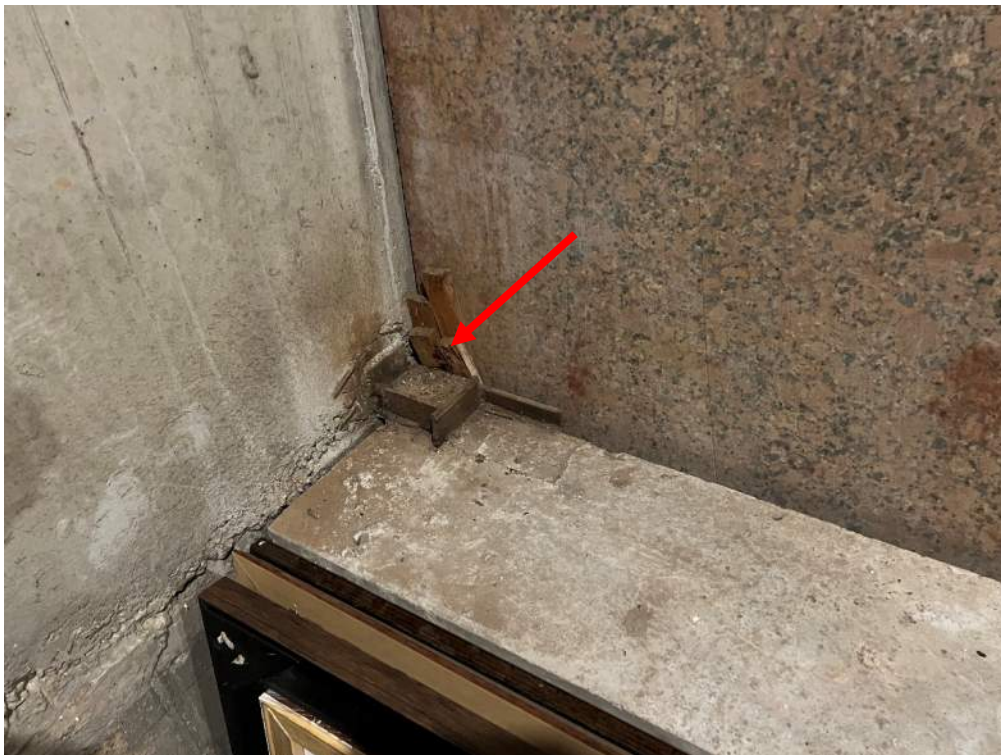
Photograph 2 – Typical gravity connection at precast concrete beam and cast-in-place concrete column supporting granite façade.
