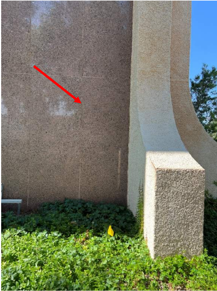
Photograph 8 - Approximate 1/8 inch lateral displacement at granite panel on south elevation.
